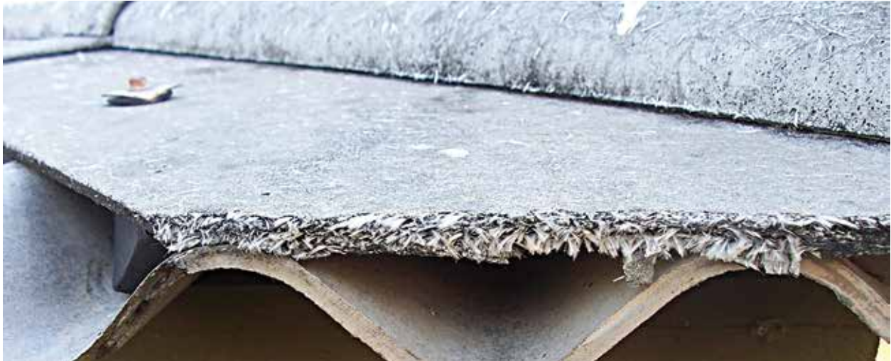
As AC roofs age and deteriorate, they will need to be replaced, raising concerns about their safe removal and disposal Photograph: Bill Bradley
