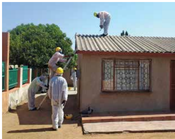
Figure 2. Bolts are loosened manually and AC roof sheeting is wetted before removal
