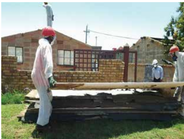
Figure 1. Asbestos contractors, wearing PPE, collect the removed AC roof sheeting before it is transported to a designated disposal site
