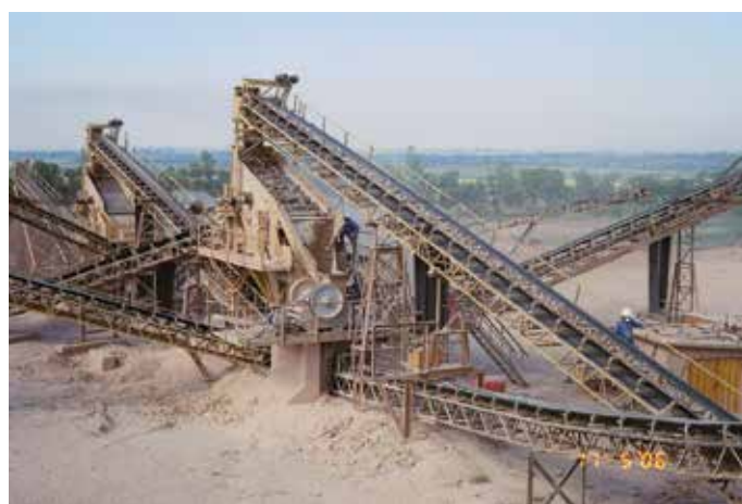
A quarry site in southern Mozambique. Employees and contractors working in this environment are at risk of exposure to respirable dust that contains silica. The dust control measures that are implemented at this operation are wetting down methods and the wearing of respiratory personal protective equipment Photo: Claudina Nogueira
